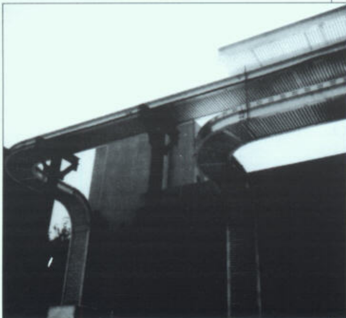
Alabama River's new system included installation of all necessary equipment, flanges, connections, fire stops, elbows, offsets, supporting structures, and other parts required to make a completely coordinated bus installation.
