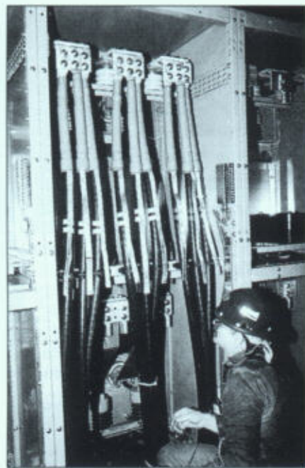
▲ Photo 11. Cables extending up from trench at switchgear terminate at the main 3000A bus. Terminations are being made up with heat-shrink termination kits and long-barrel, double-hole, copper compression connectors. Flat copper braid from each conductor has not yet been connected together and grounded to grounding bus in the switchgear.
