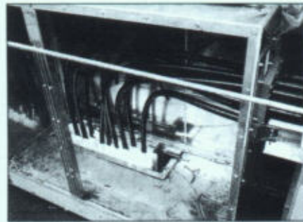
▲ Photo 8. Typical pullbox is about 5 \times 4 \times 4-ft. Cable bus conductors enter at right through an environmental seal; then electricians carefully feed cable down to teams of electricians at various levels in the motor room. The nine conductors are arranged in a parallel arrangement to enter a 36-in wide vertical cable bus tray going down to the motor room. Grounding conductor from cable bus connects to the box and continues down to the vertical cable bus tray.
