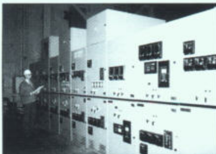
◀ Photo 12. New 7.2kV-rated, 3000A switchgear in center of motor room is being checked by Bill Pruss, U.S. Steel. (Heat-shrink terminations are being installed on opposite side). Cubicles contain 1200A vacuum circuit breaker that supply unit 6.9kV/480/277V substations, 6.9kV rolling mill motors, huge motor-generator sets, or rectifiers that supply DC power for DC rolling mill motors.
