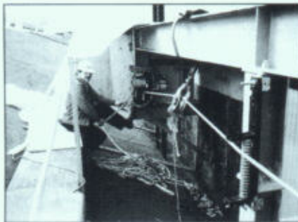
▲ Photo 7. Pulling winch mounted several feet beyond end of last roof-mounted pullbox provides the power to pull the cable from the ground-located reel. Pulling rope, which is \frac{3}{4} in. dia, travels over vertical rollers mounted on steel in foreground and sheave near winch.
