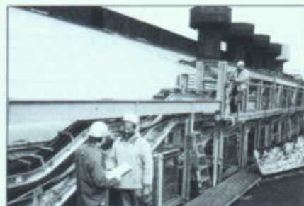
▲ Photo 5. Three-stack cable bus running along the roof area comes from the vertical tower in background. Note that the top cable bus has all nine cables in place. Only the top cover remains to be installed. Just below, support blocks are installed in bottom sections, and the first cable is in process of being pulled into place. Note, behind ladder, how stacked cable bus peels off vertically into pullboxes for descent into plant motor room.
