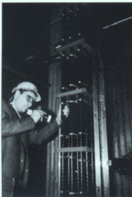
▲ Photo 10. Alan Patton, electrical engineer for Chapman Corp, inspects cable bus near floor just before it enters trench that extends to a 7.2kV-rated switchgear in the center of the motor room. The trench, which runs along the length of the switchgear, is 2 ft wide and was cut out of 20 in. thick concrete floor.
